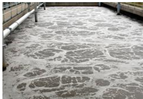
2b: Aeration tank in operation
